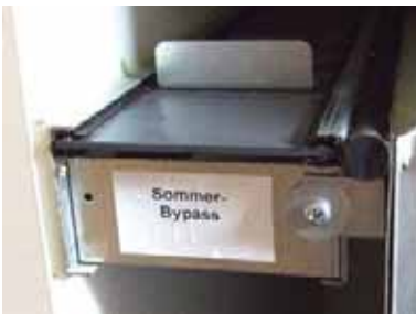
The sommer-bypass can be used for cooling in the summer if needed. Source: MosArt Architecture.
