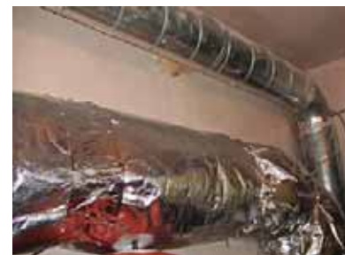
Supply air ducts should be well insulated. Source: MosArt Architecture.
