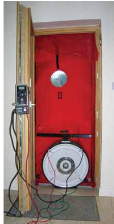
No more than 0.6 air changes/hour at 50 Pascal pressure should be observed in accordance with the Passivhaus Standard. This should be checked for compliance with a blowerdoor test which will immediately highlight leaky areas. Air-tightness can be achieved through the use of membranes, roofing felts and plasters combined with sealants and vapour diffusing resistant materials. Source: UCD Energy Research Group.
