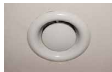
Ceiling air supply vent. Source: MosArt Architecture.
